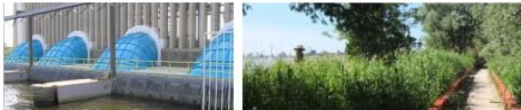
Pumping stations + green embankments
